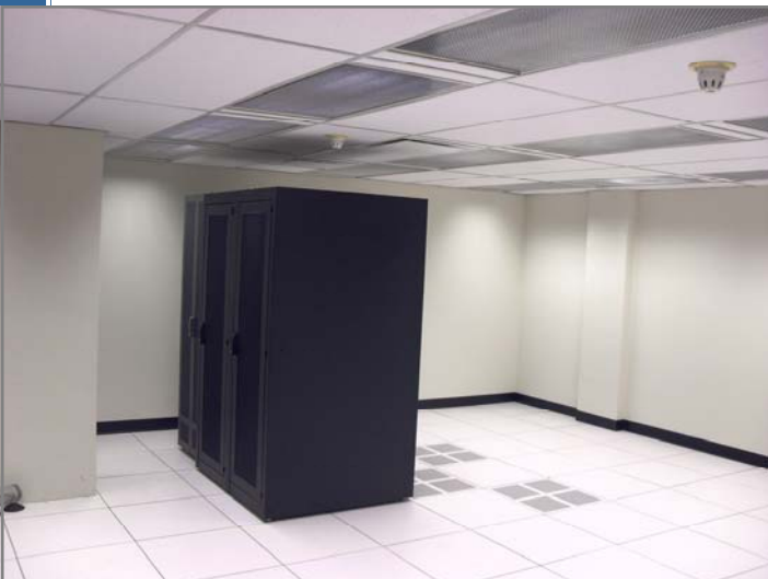
Building 20—2nd Floor Colocation Room
